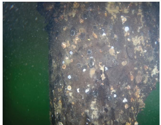
Image left and right: Rot, Marine borer and aggressive marine environment have continued to eat away at the structural supports
