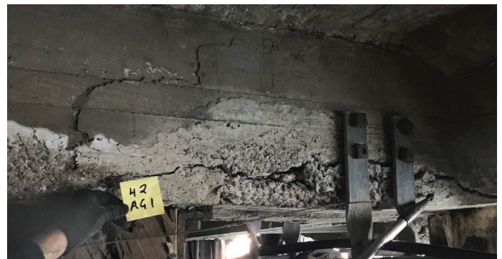
Beam cracking Wharf 14
