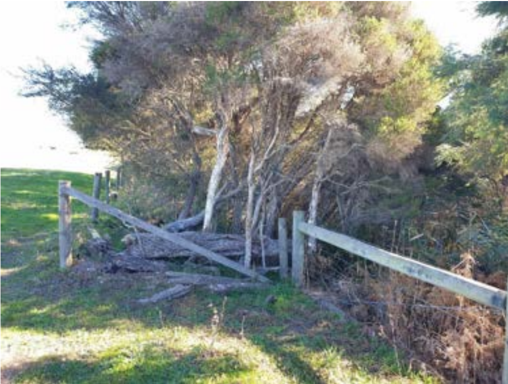
Photo 5 Fence damage observed along southern boundary of offset site, 22 May 2024
